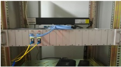
Subway base station(FTU field management unit) ↓
