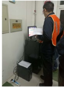
Beijing subway line 4 OMC ↑ leaky cable monitoring system
